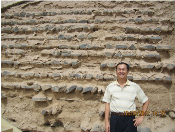
Fig. 6 A close look of Reinforced Great Wall in Black Mountain: the wall was built with loess sandwiched by rock pieces (spacings of reinforcement are about 40 cm)
