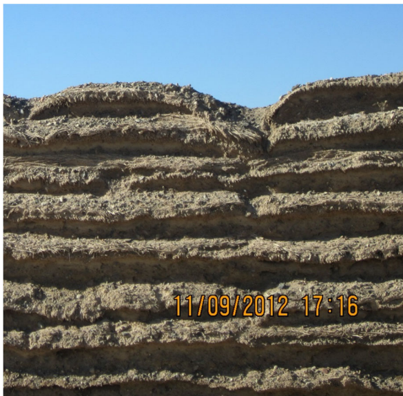
Fig. 3 A close look of a profile of the Reinforced Great Wall of the Han Dynasty in Yangguan Pass (spacing of reinforcement is about 40 cm)
