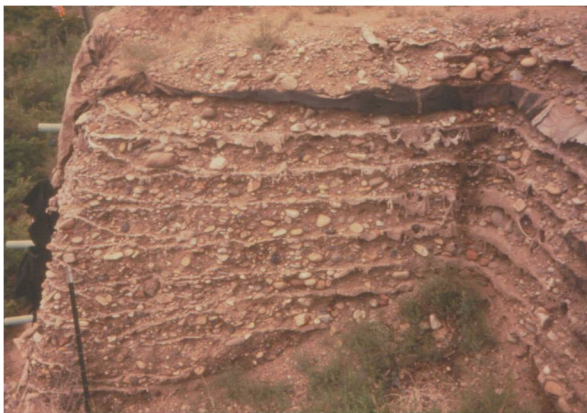
Fig. 14 A cut of the Glenwood Canyon geotextile test wall along I-70 (the front-facing was removed, but the wall has been stable for many years before demolition)
